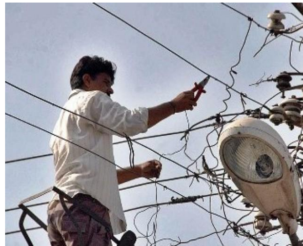
Figure1: Tapping electricity directly from the distribution feeder -bypassing the meter.
