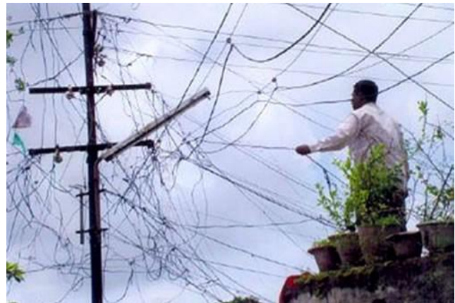
Figure1: Tapping electricity directly from the distribution feeder -bypassing the meter.
